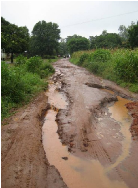
The state of the main road to the hospital
